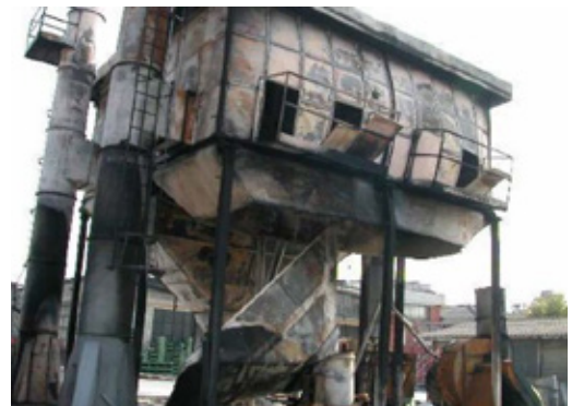
Dust Collector After Explosion
