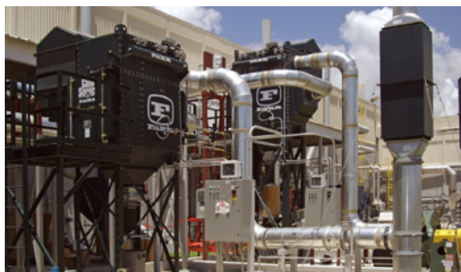
These dust collectors are equipped with passive and active controls that include an explosion vent and ducting, as well as a chemical isolation system mounted on the inlet duct.
