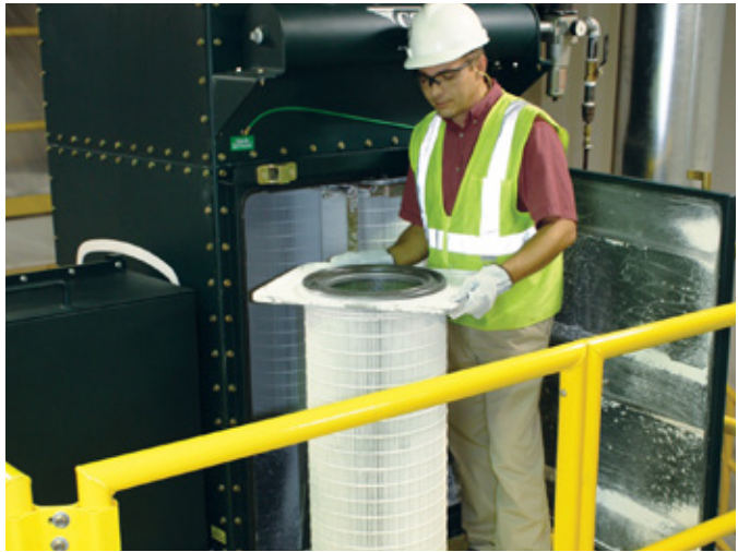
Figure 5: Vertically-mounted dust collector filters
