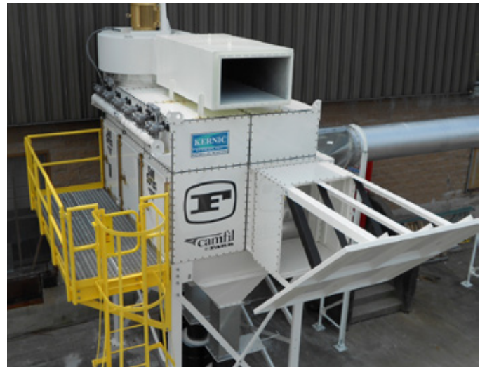
This dust collector is equipped with an explosion vent with vertical upblast deflector plate. Other safety features include a sprinkler system and filters with special carbon-impregnated media for static dissipation.
