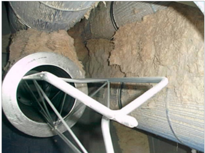
Figure 6: Horizontally-mounted dust collector filters
